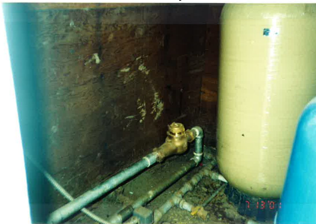
Flow Meter Inside Well House
