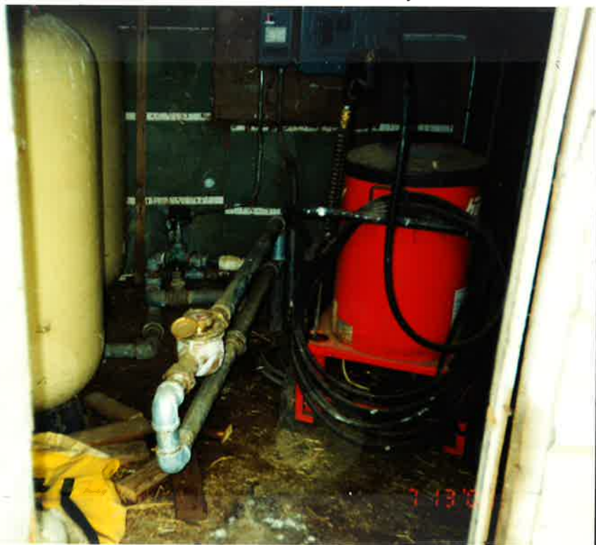
Flow Meter In Well House
