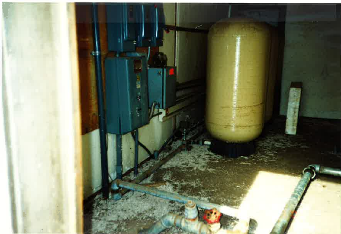
Pressure Tanks For Well #3, Controls For Wells 3 & 4
