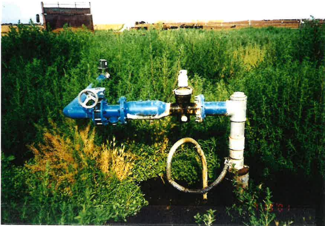
Figure #1: The well and mainline (WMIS #400072, Well Tag A0011455)
