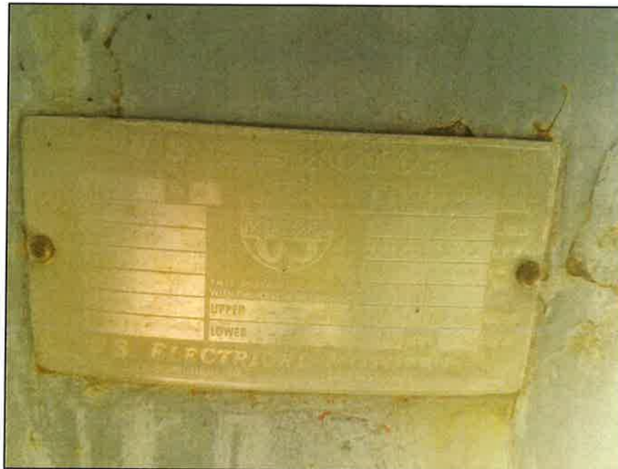
Figure 10: Well 5 motor nameplate.
