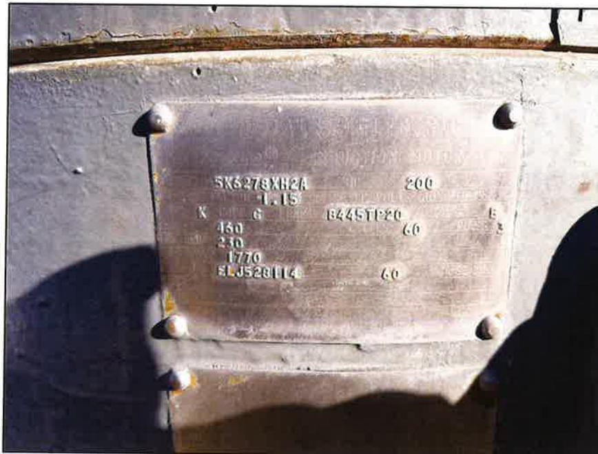
Figure 12: Well 6 motor nameplate.
