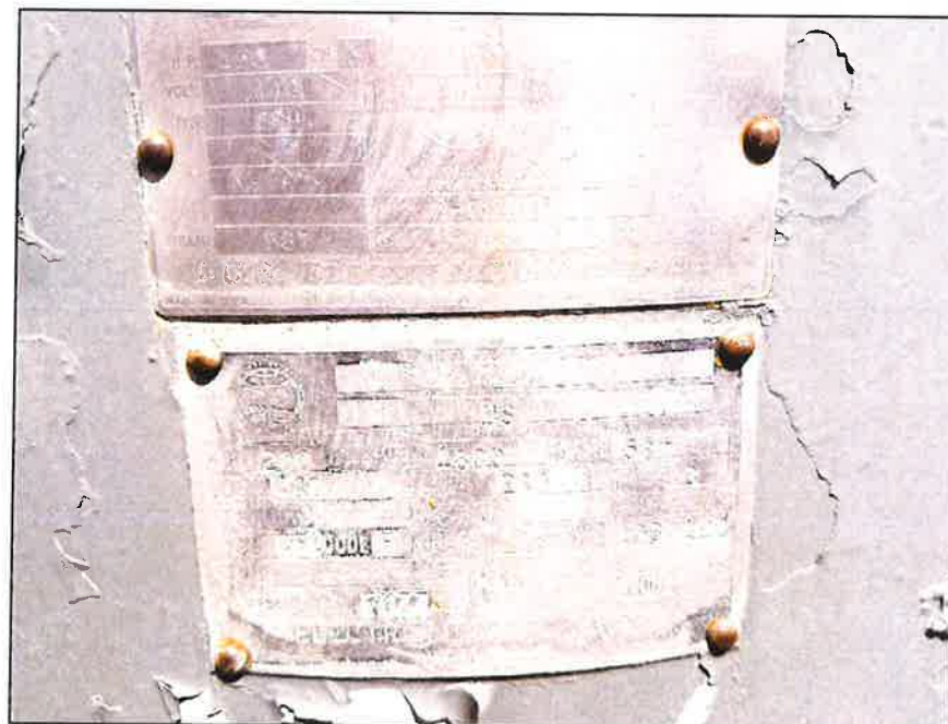
Figure 6: Well 3 motor nameplates.
