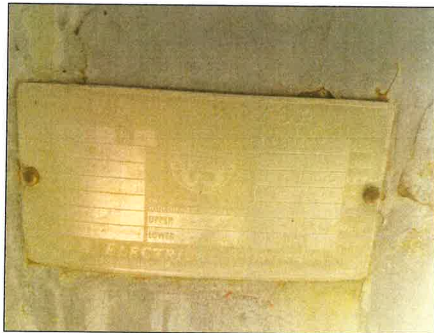
Figure 10: Well 5 motor nameplate.
