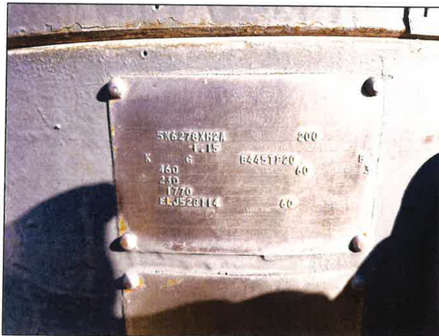
Figure 12: Well 6 motor nameplate.
