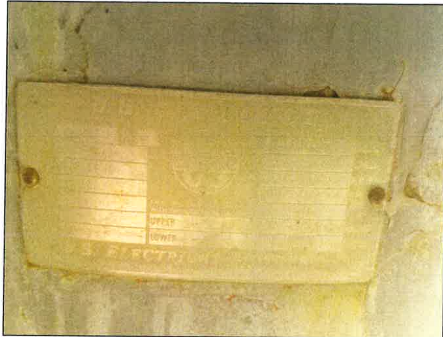
Figure 10: Well 5 motor nameplate.
