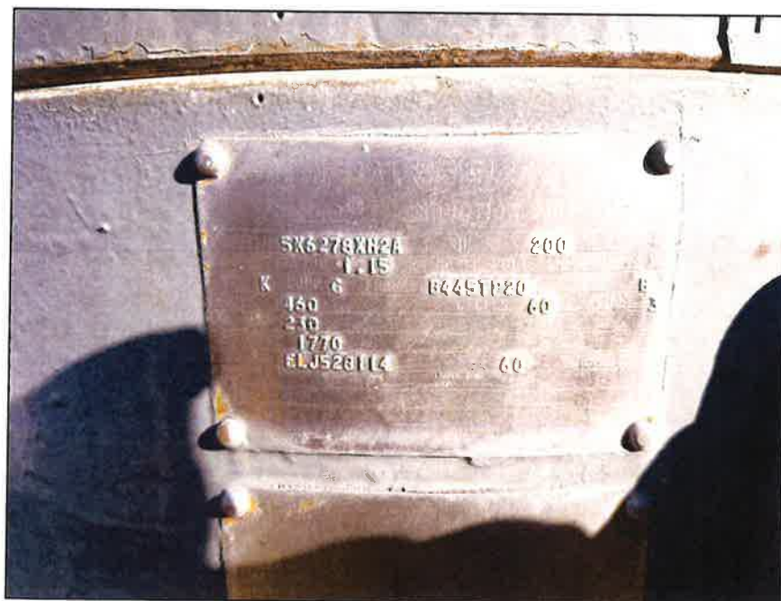
Figure 12: Well 6 motor nameplate.
