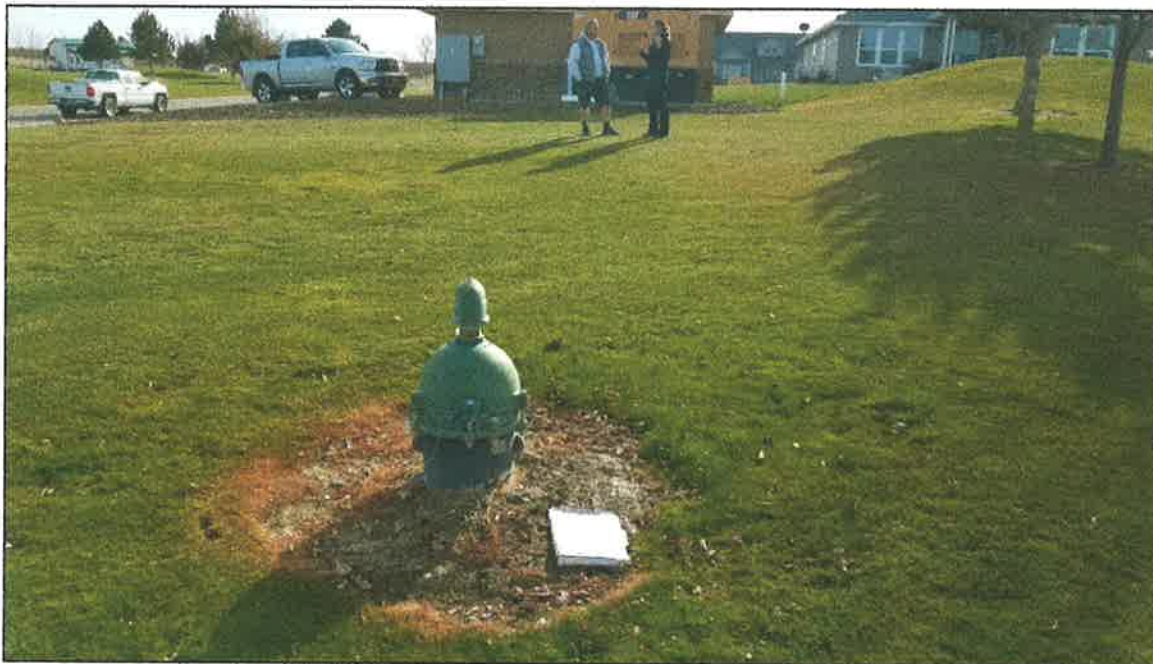
Figure 1: Well 2 in foreground with Well 1 in background, near the backup generator (almost hidden by operator's left leg).
