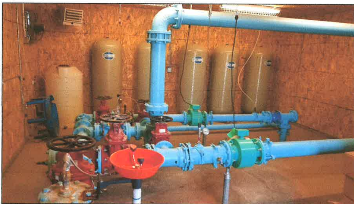
Figure 2: Well house mechanical piping. Well 1 6-inch flowmeter (green) in foreground with Well 2 4-inch meter closer to pressure tanks.
