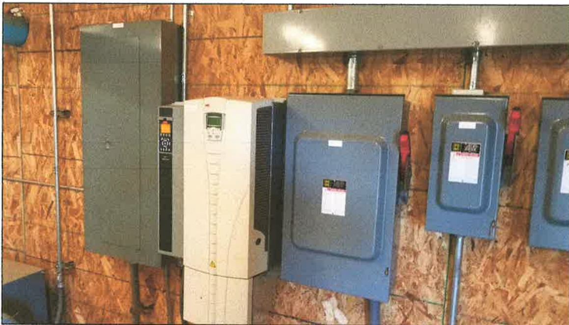
Figure 4: Both pumps are equipped with variable speed drives.
