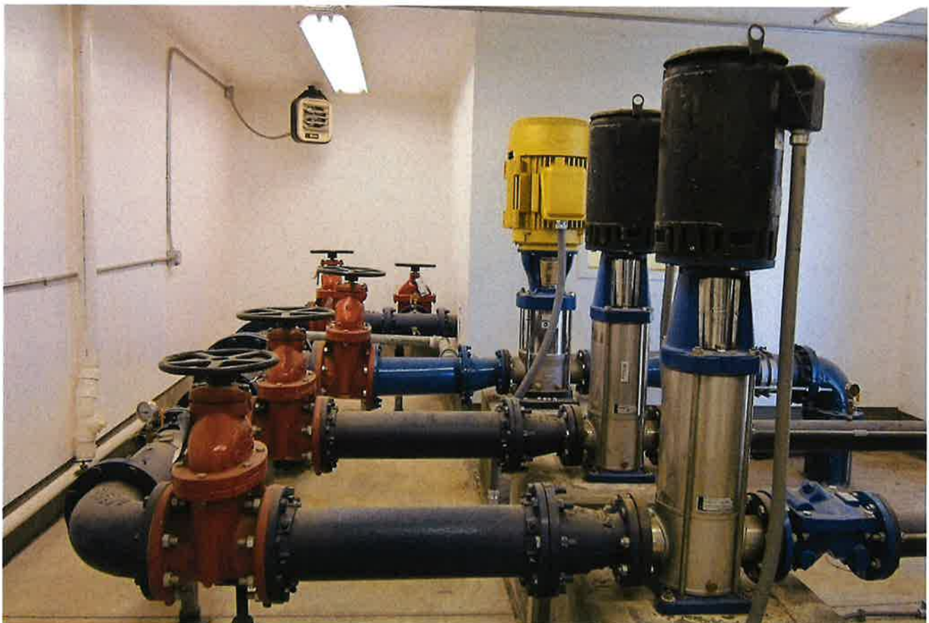
Below: Existing well booster pumps system
