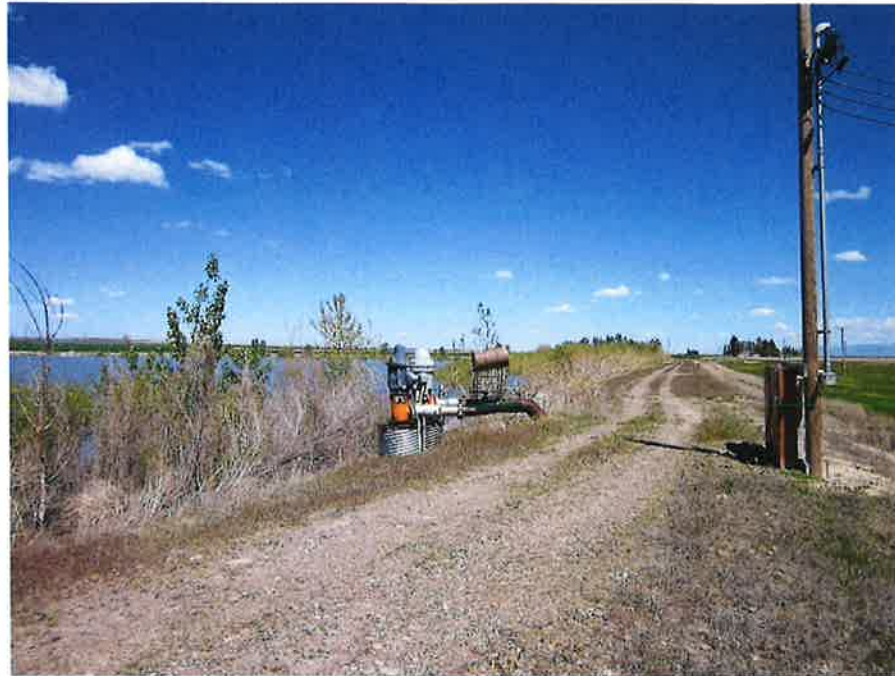
Figure 5: East reservoir pumping station
