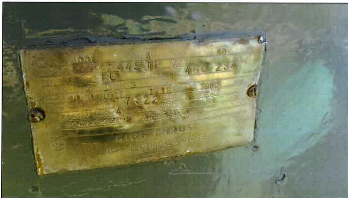
Figure 6: Section 20 motor nameplate.
