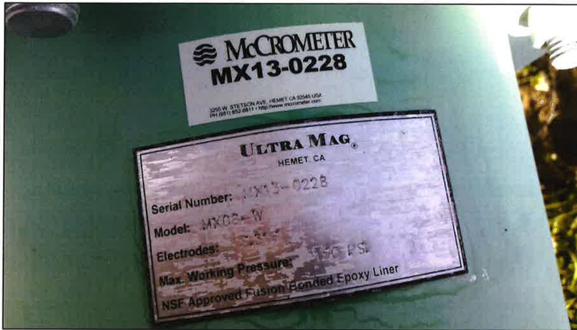
Figure 3: Section 29 flowmeter nameplate.
