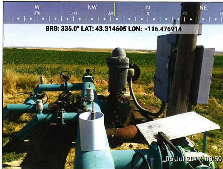
Figure 5: Section 20 well and plumbing network. As noted in exam report, booster pump in photo lower right is no longer used. When it was used, it boosted pressure from water stored in the adjacent pond.
