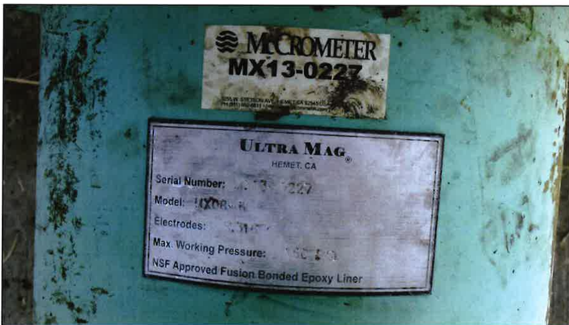
Figure 8: Section 20 flowmeter nameplate.
