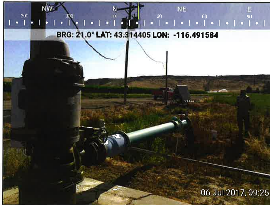
Figure 1: Section 29 well with flowmeter installed in discharge pipe.
