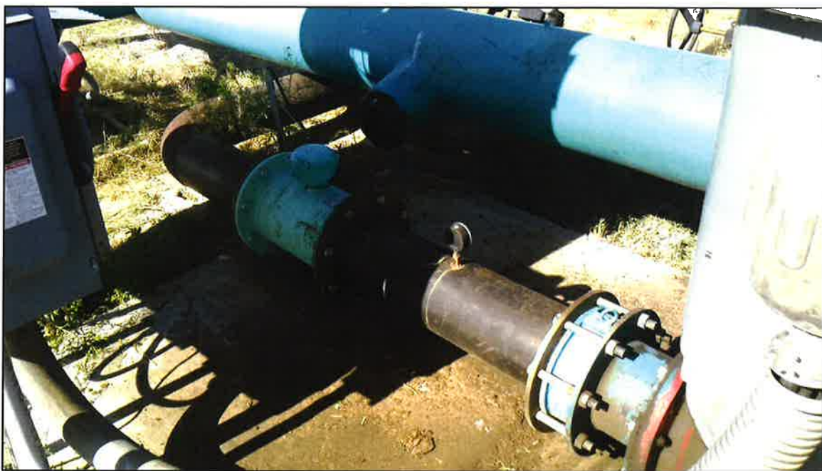
Figure 7: Section 20 flowmeter installed in discharge pipe.
