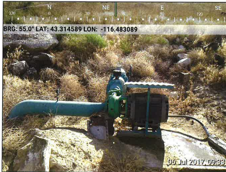
Figure 9: 50-hp booster pump.
