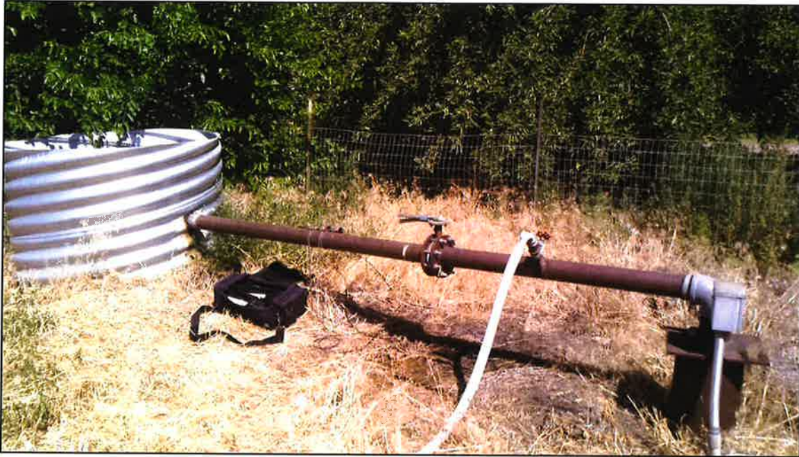
Figure 1: Well is equipped with a submersible pump and 4-inch diameter steel discharge pipe.
