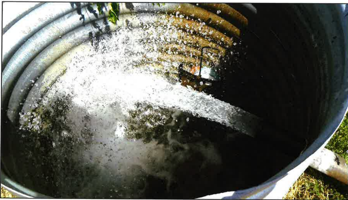
Figure 2: Well discharges into a CMP sump where it then flows by gravity to Pond A (see map).
