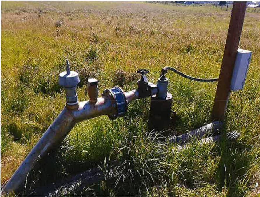
A 10-hp submersible pump diverts water to a 6-inch mainline at 65 psi operating pressure.
