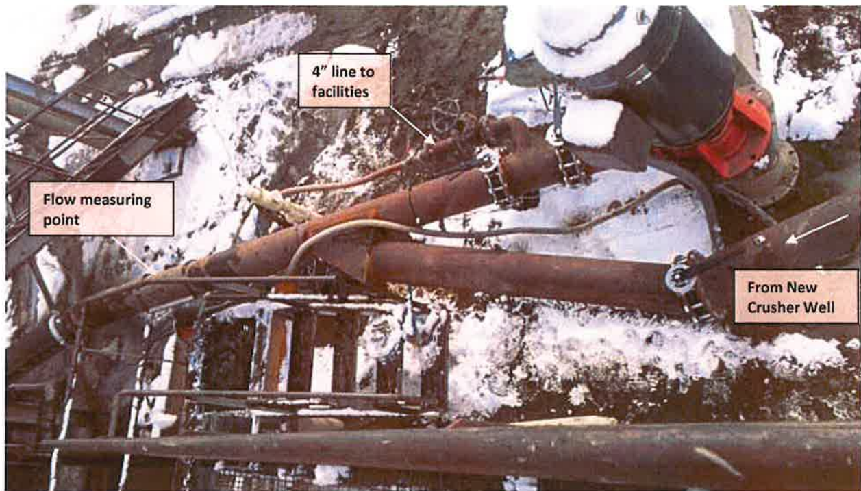
Overhead view of piping
