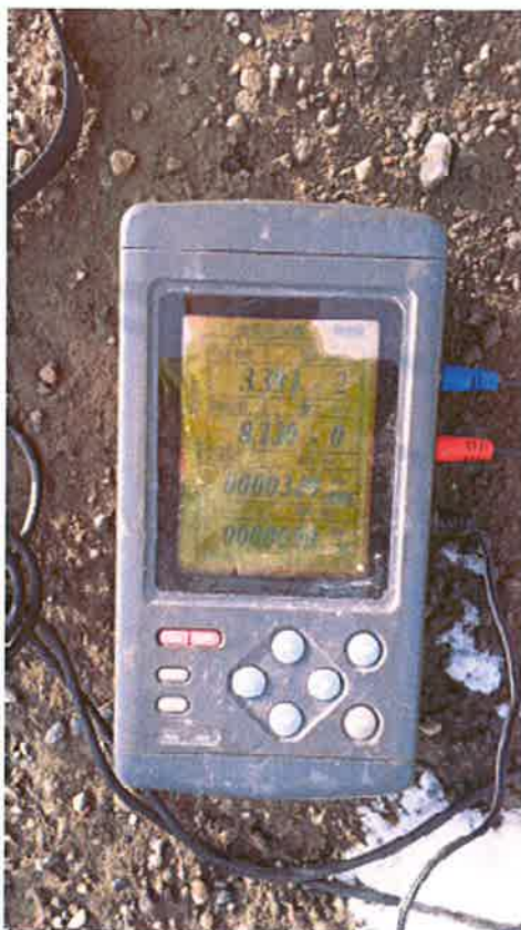
Flow meter readout for condition #2 in the 4" line
