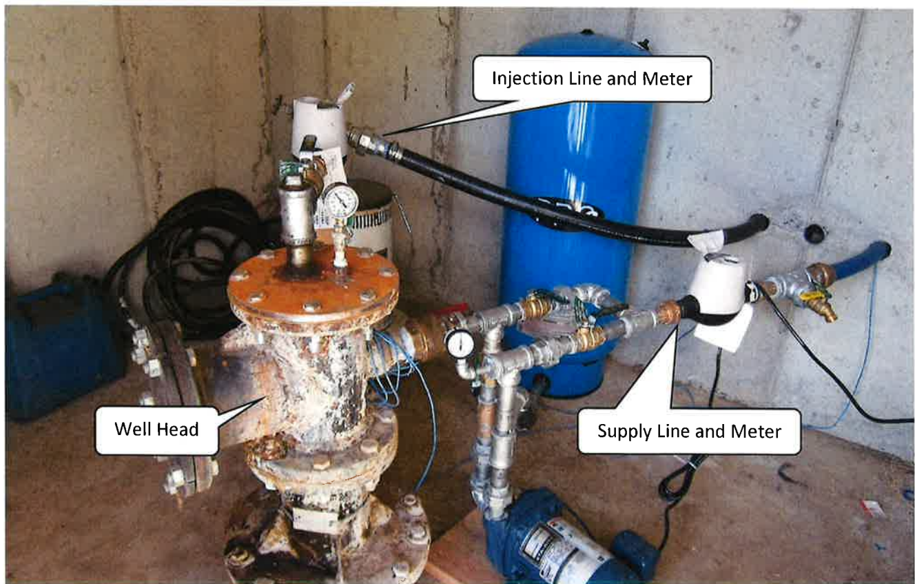
Below inside well house: Geothermal well, flow meters, supply, and return lines
