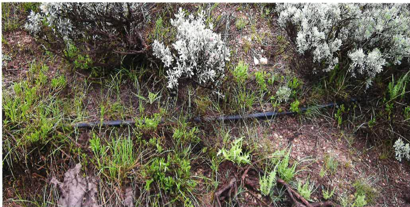
Above: Pipe to Trough from Spring #1
