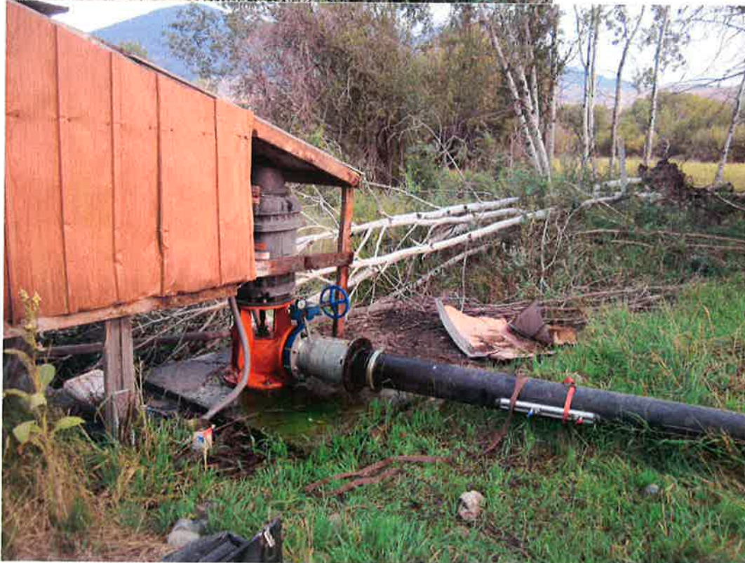
Pump: The pipe flows west up hill
