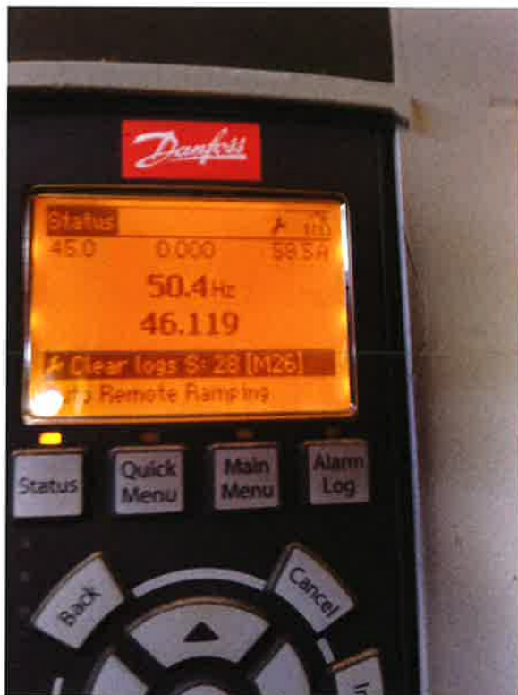
The motor is driven by VFD. The motor runs at roughly 50 hz frequency to maintain a pressure of 65 psi while watering using the wheel line.
