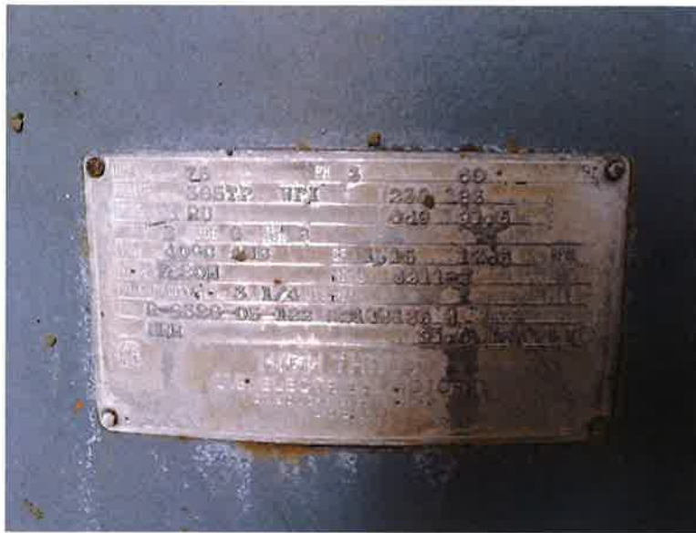
The motor specification plate shows the motor is a 75-hp motor by US Electrical
