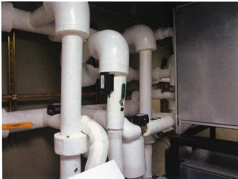
More plumbing with two heat pump units at right. All piping is well insulated.
