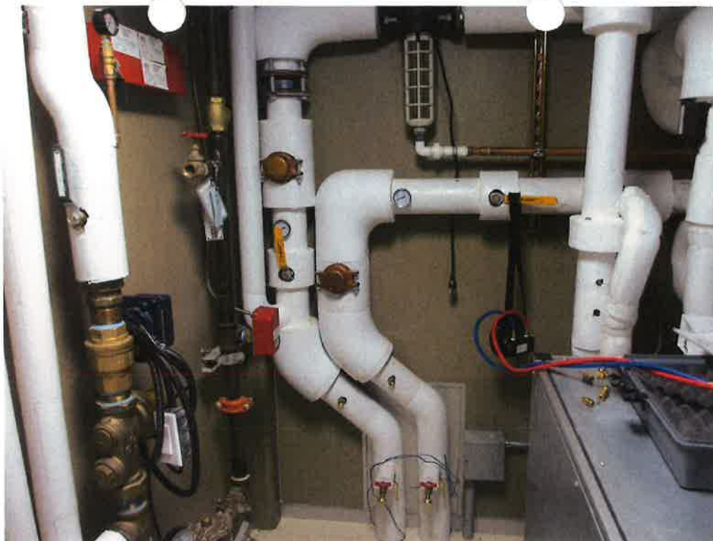
Plumbing inside the mechanical room. Heat pump unit at lower right.
