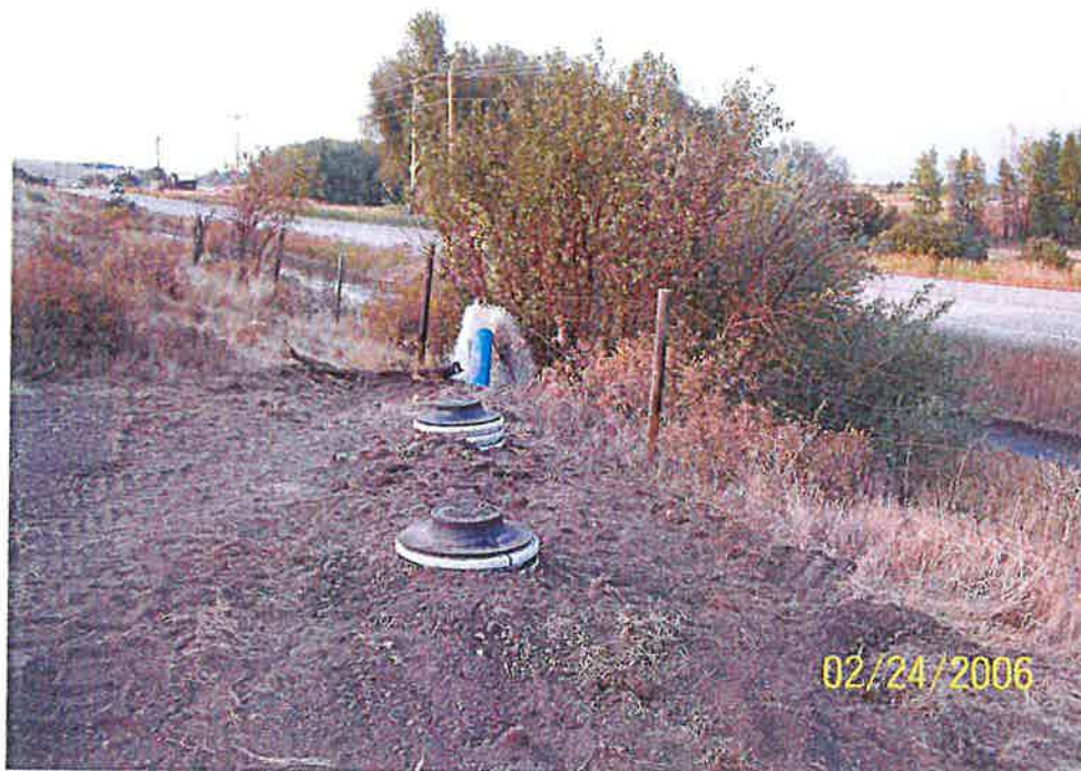
Terminus of the Sam's Hollow mitigation pipeline.
