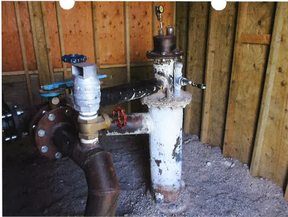
Point of diversion and associated plumbing inside well house.
