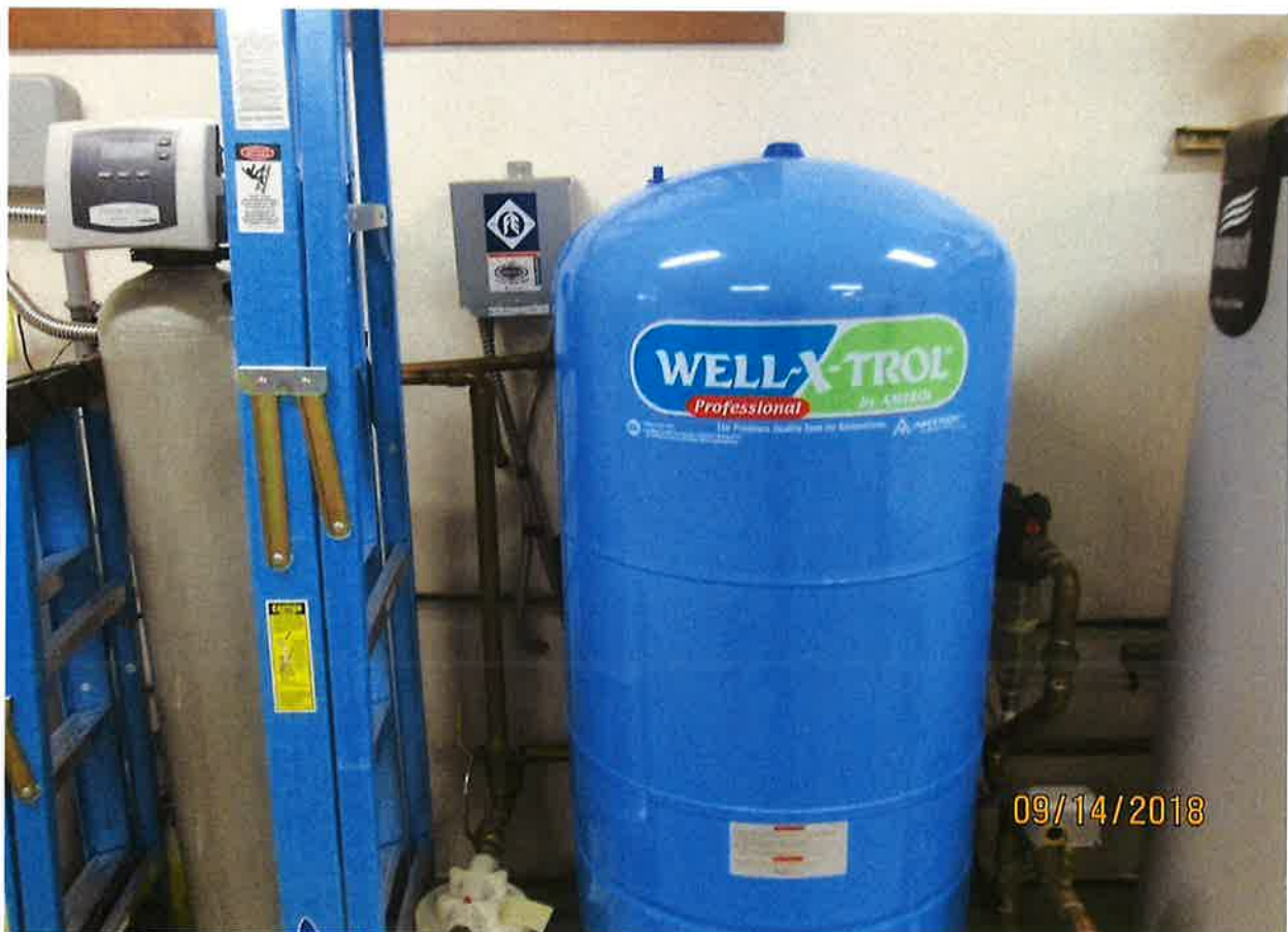
Unable to perform flow measurement because of buried pipes to pressure tanks.
