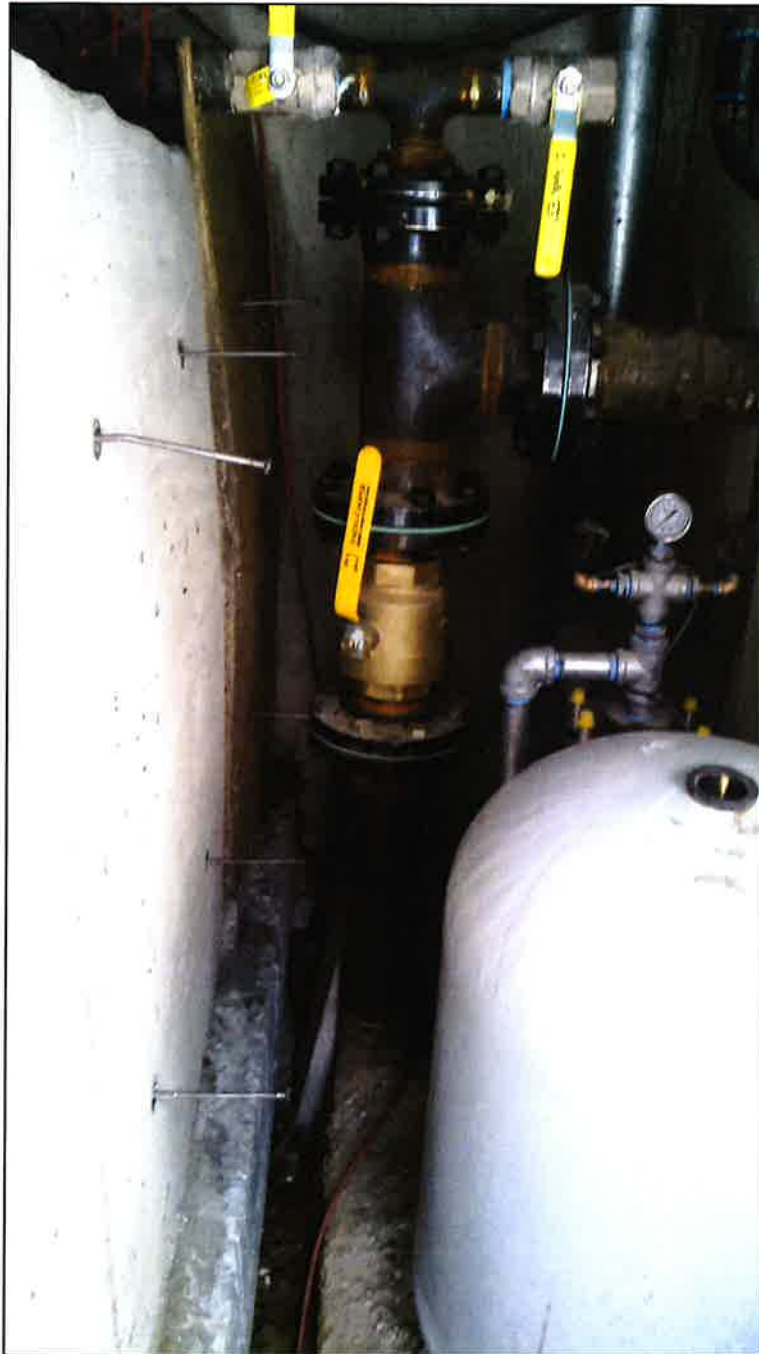
Figure 6: Mechanical piping from pond pump in distillery. Flow enters from pipe up through floor.
