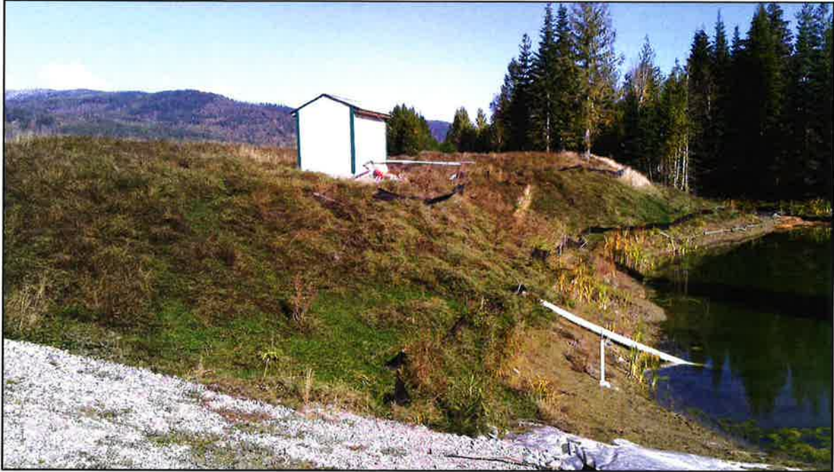
Figure 1: Pumphouse and pipe into pond for submersible pump.
