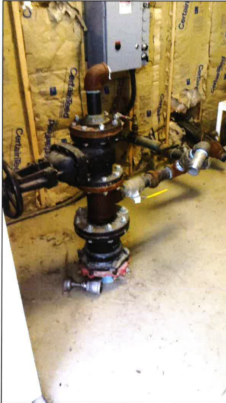
Figure 5: Pump house mechanical piping. Flow enters from pipe on far right, can discharge back to the pond (pressure relief) through middle pipe, and flows to the distillery on left pipe, down through the floor.
