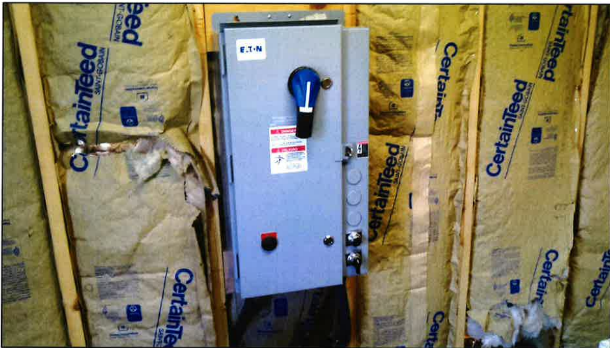
Figure 4: Pond pump controls.
