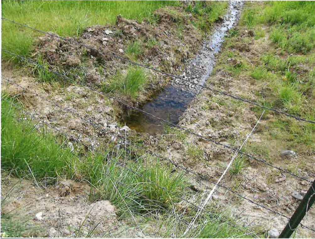
Figure 1. Pont of diversion. Culvert carrying waste water from neighboring property crosses under road and enters a ditch on the Junayo Ranch property.
