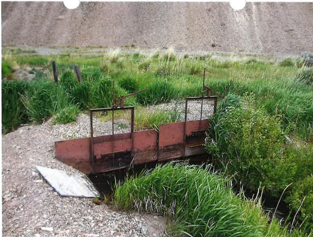
Lower POD- French Creek through left headgate, Ogden through right.
