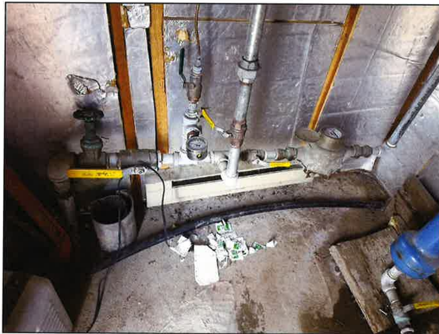
Figure 2: Well 2 mechanical piping including Sensus flowmeter.
