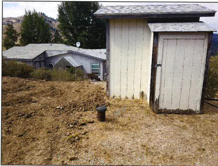
Figure 6: Well 2 mechanical piping including Sensus flowmeter.
