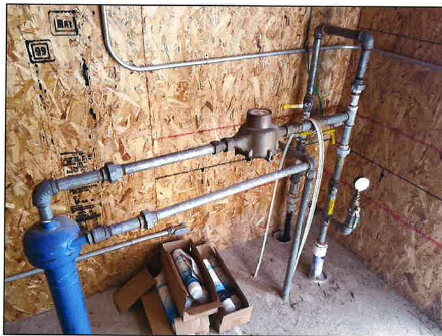
Figure 7: Well 4 mechanical piping.
