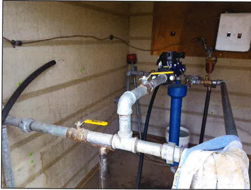
Figure 5: Well 3 mechanical piping.
