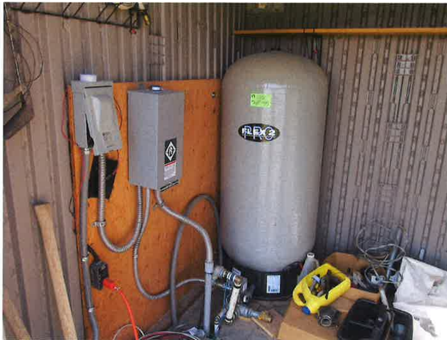
Figure 3. Inside of pump house showing pump controls and pressure tank.
