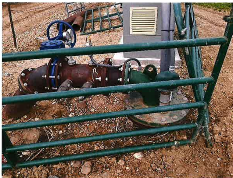
12-inch well with 16-inch flanged head. 125 hp pump. 80 psi.
