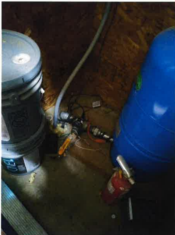
Figure 4 The domestic and commercial supply line goes into this 81-gallon pressure tank for use in the barn and the tasting room.
