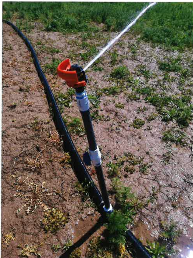
Nelson R33 Rotator sprinklers used to irrigate the southern pasture of the place of use.
