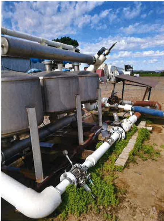
The location where the mainlines from the two wells come together and pass through the flow meter.
