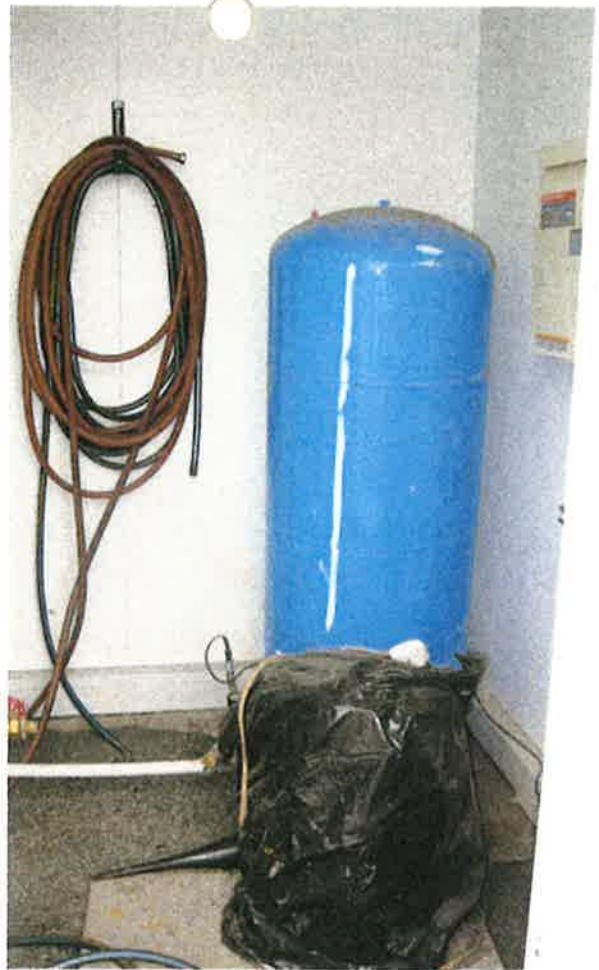
Interior Manifold BLDG
