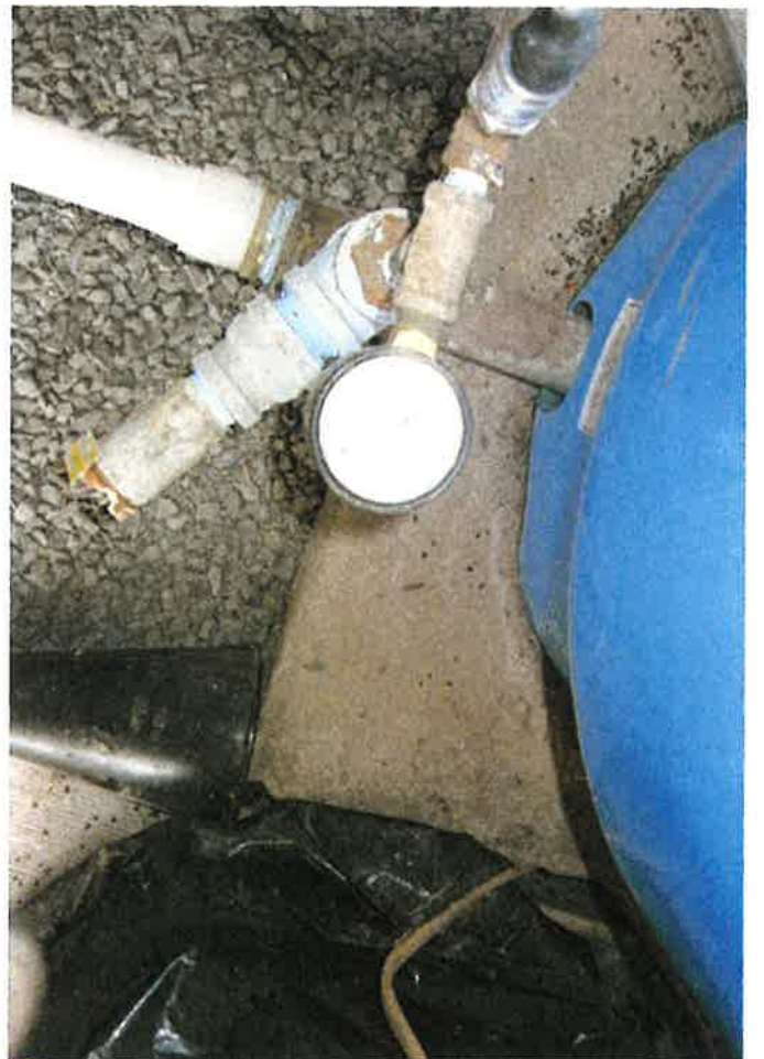
Gauge Interior Manifold BLDG
