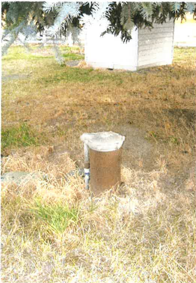
Well and Manifold BLDG
