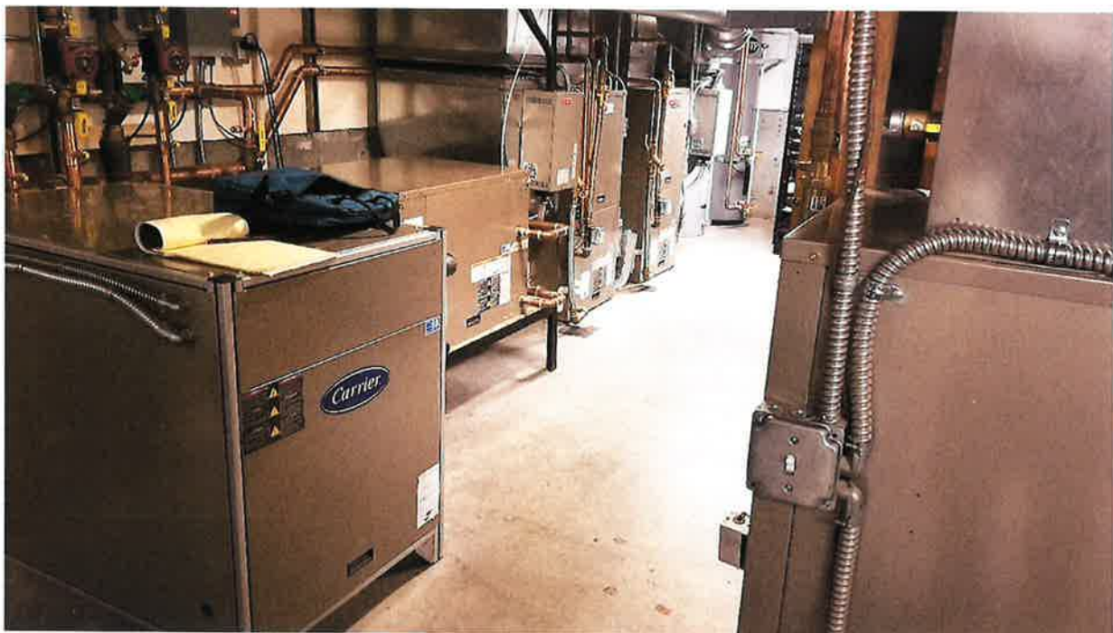
Figure 6: Five of the Eight Heat Pumps
