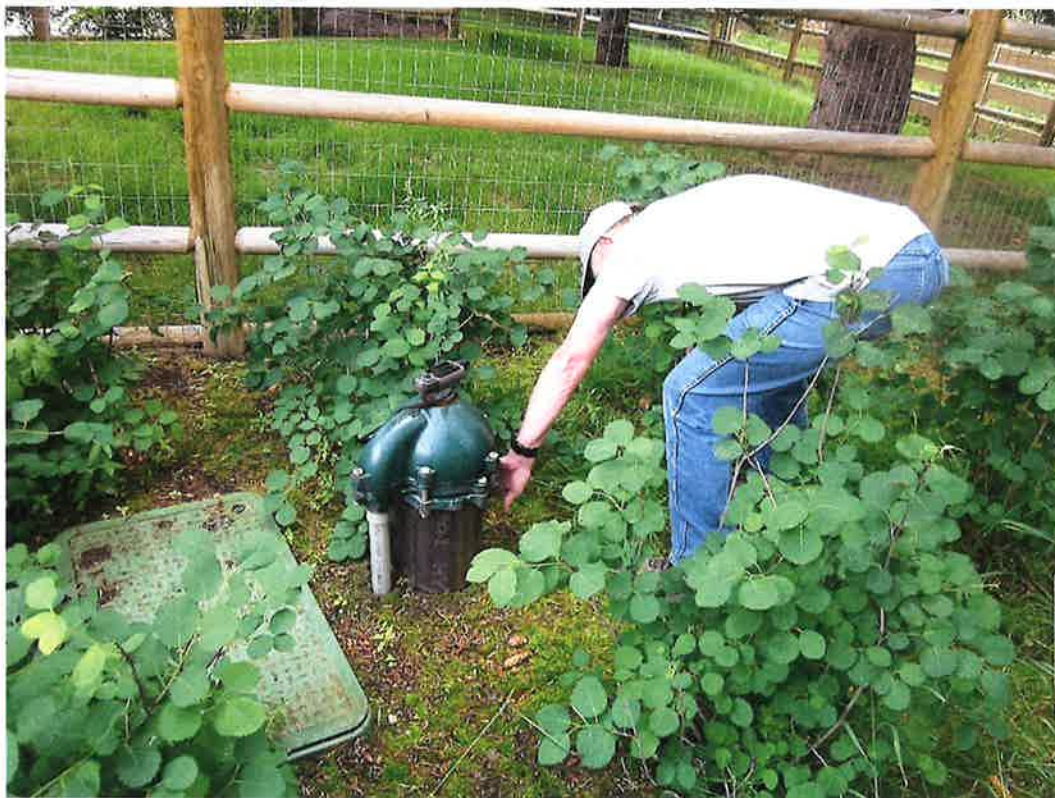
Figure 2: Well Head (South Side of Home)
