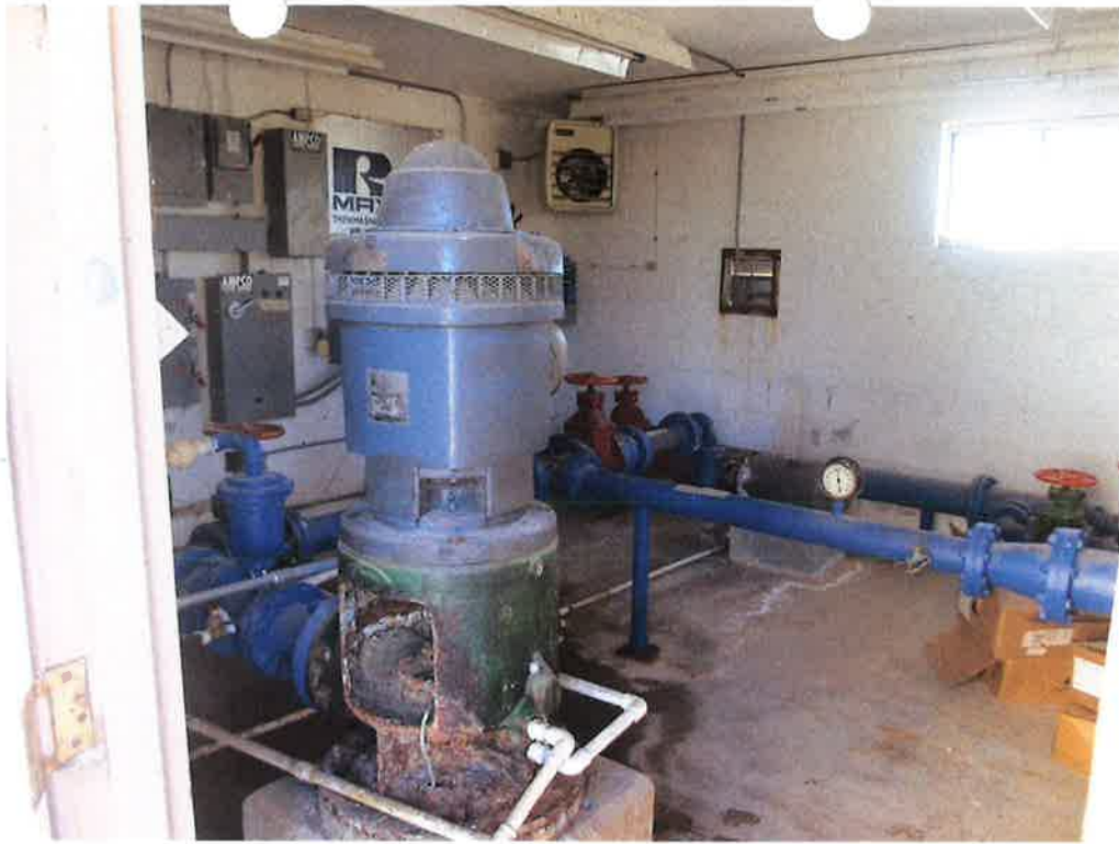
Well #1 and plumbing inside well house
