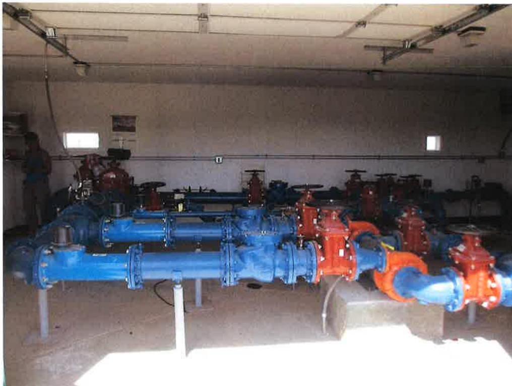
Plumbing inside Well #3 well house
