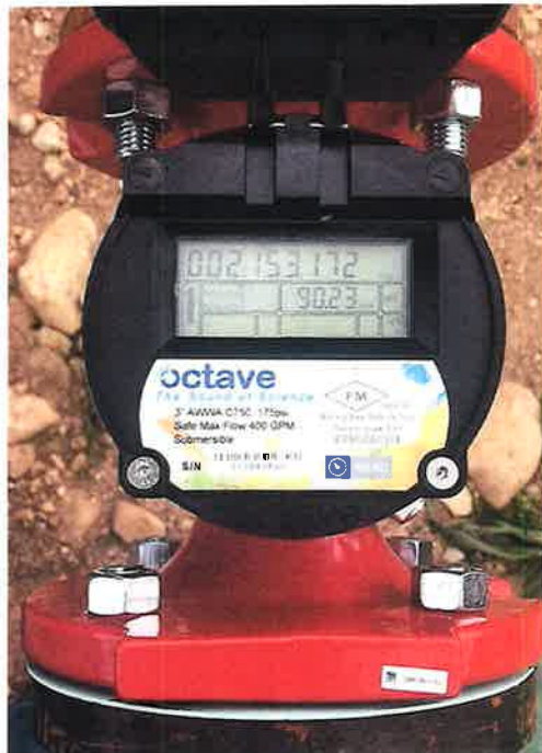
Installed System Meter
