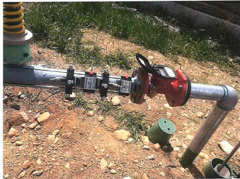
Installed flow meter
