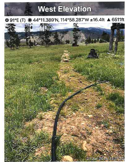
Three inch sprinkler line
