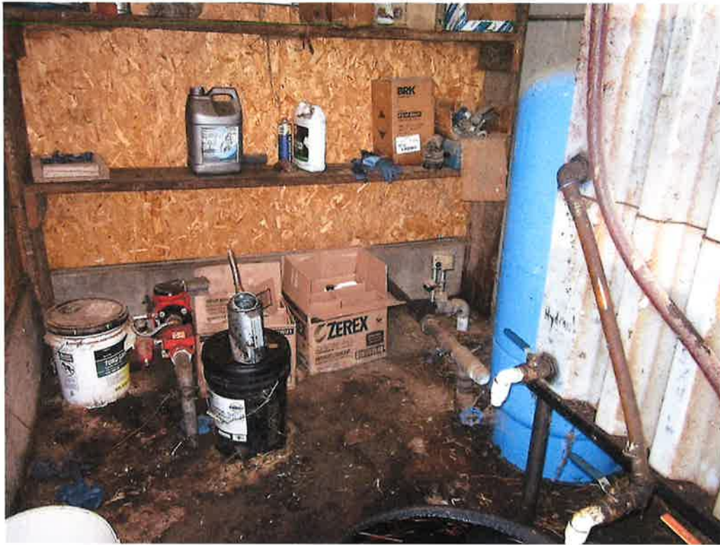
Figure 3: Inside pump house
