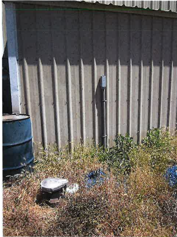
Figure 1: Well head & Pump House
