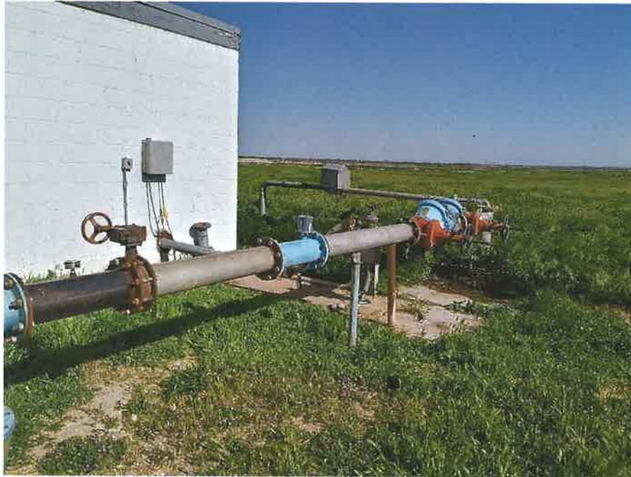
The mainline from the well (and the wastewater supply line) which has the inline-flow meter.
