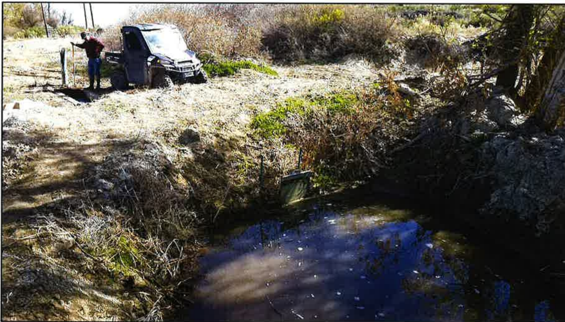
Figure 2: Diversion with headgate in foreground and flume with trash rack in left background.
