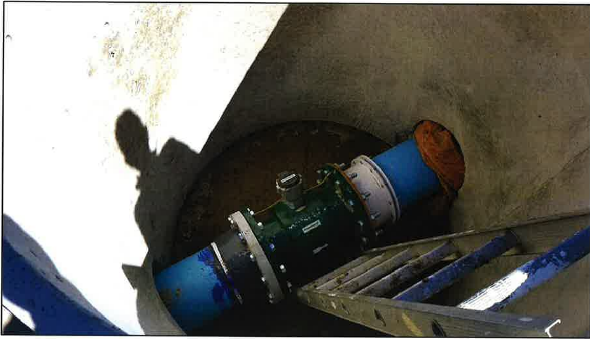
Figure 5: Magnetic flowmeter installed in a concrete culvert vault.
