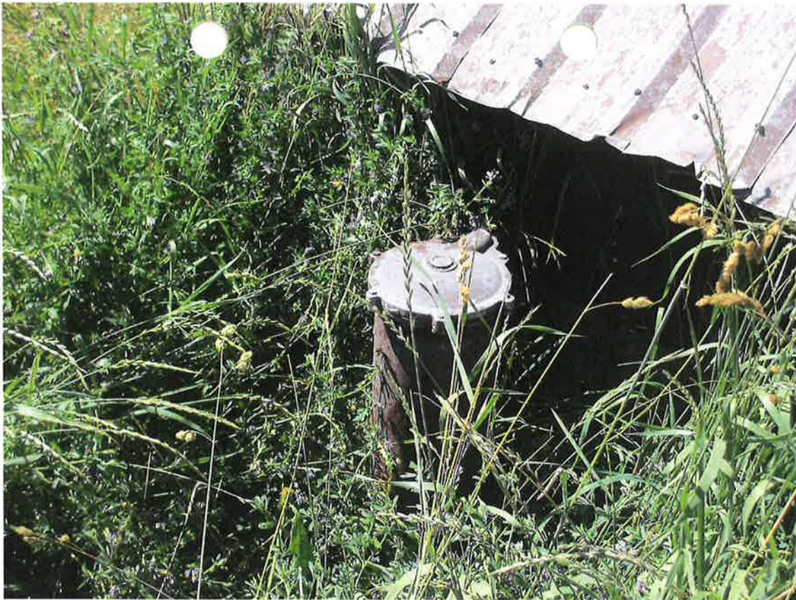
POD- irrigation well on Roskelley property.
