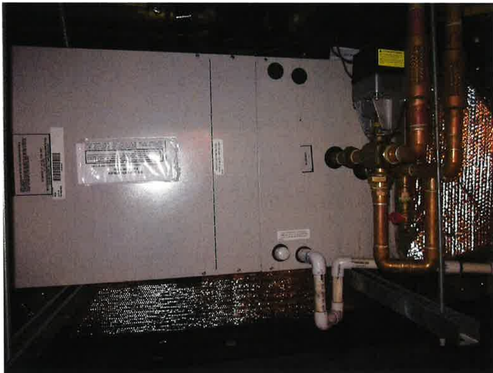
Figure 4: One of the eight heat pumps
