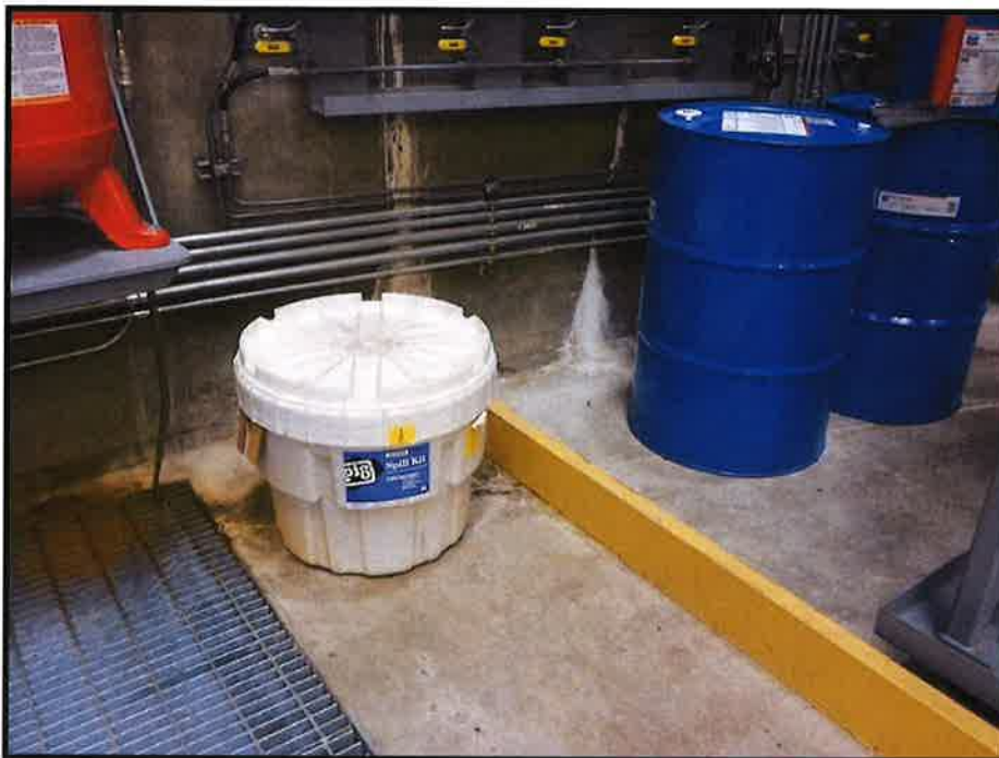
Photo 7. Arrowrock spill kit and secondary containment around oil drums.
