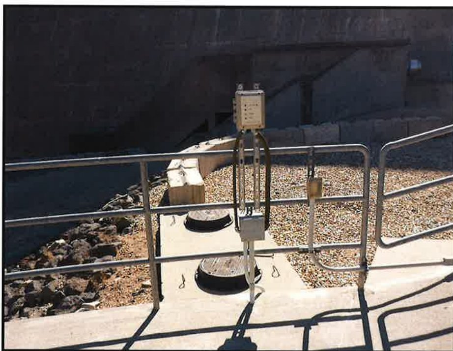
Photo 8. Oil and water separator control on powerhouse deck.
