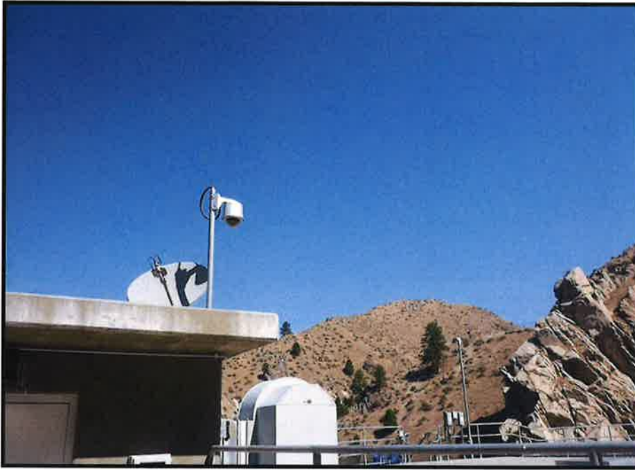
Photo 5. Security camera on powerhouse.
