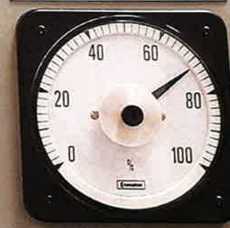
• WICKET GATE POSITION •
