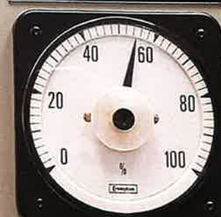
• WICKET GATE POSITION •
