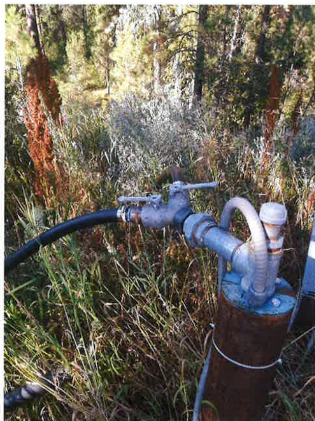
The six-inch well with a two-way valve that diverts water to separate mainlines.
