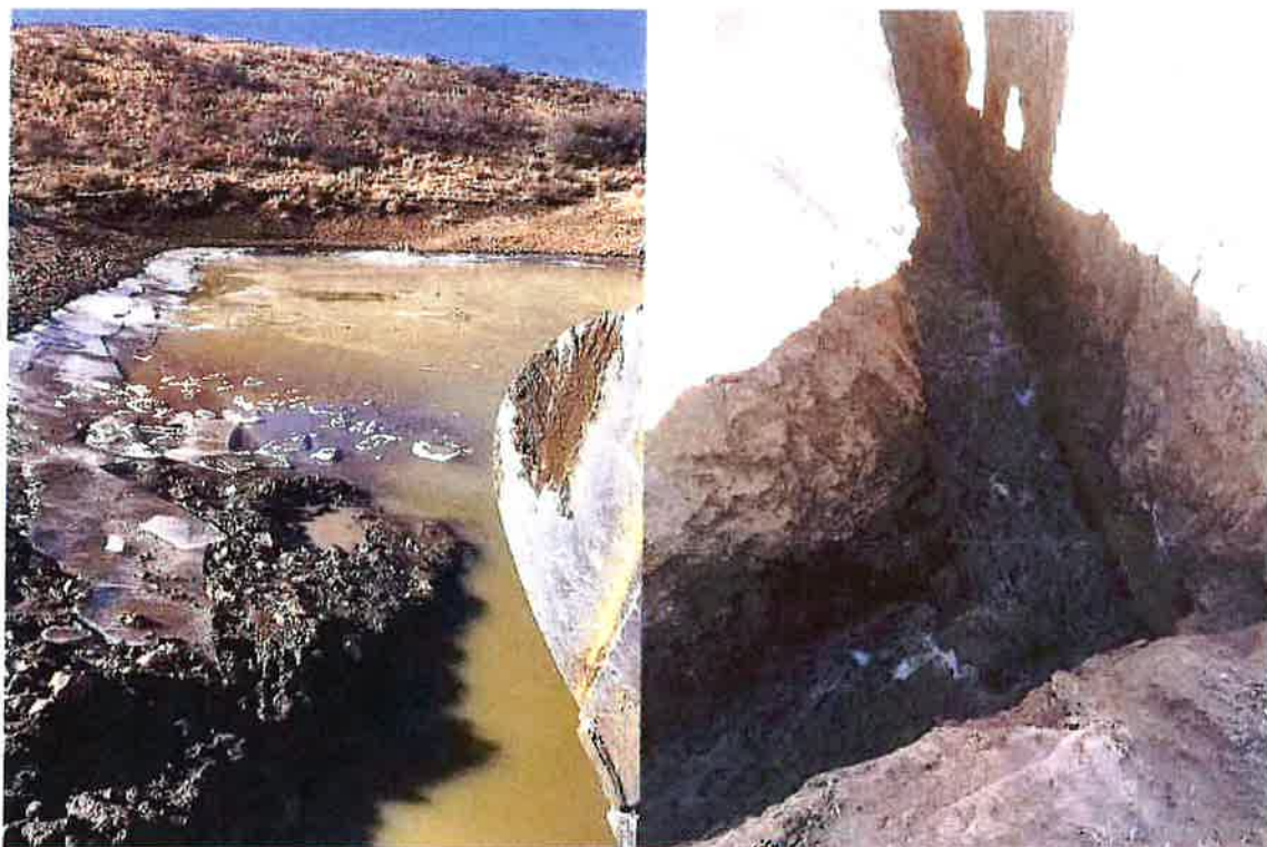
Photo 3: Photographs documenting Pond No. 11 breach; submitted by Rockford Stone (contractor).
