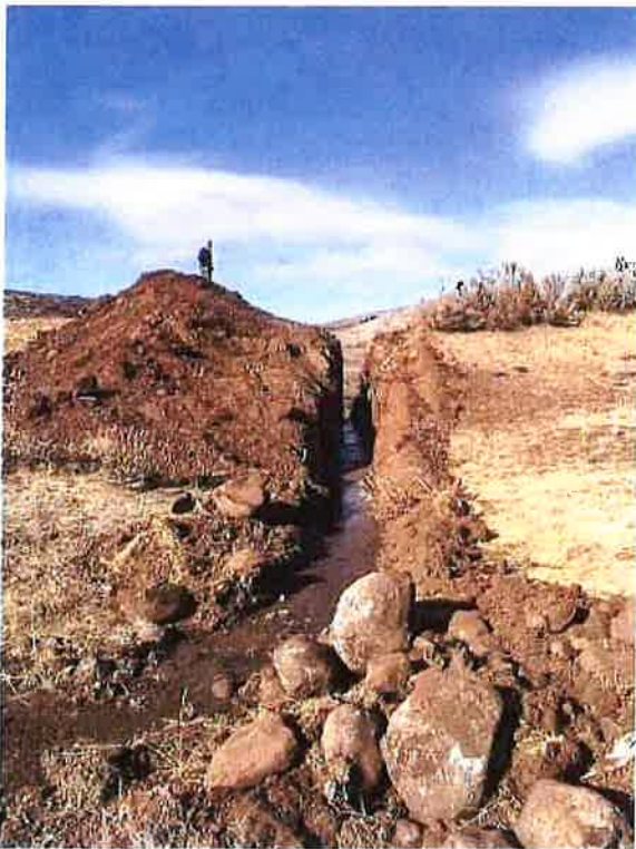
Photo 2: Photograph documenting Pond No. 4 breach; submitted by Rockford Stone (contractor).
