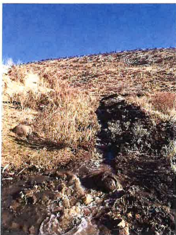
Photo 4: Additional photograph documenting Pond No. 11 breach; submitted by Rockford Stone (contractor).
