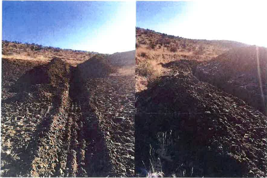
Photo 1: Photographs documenting Pond No. 3 breach; submitted by Rockford Stone (contractor).
