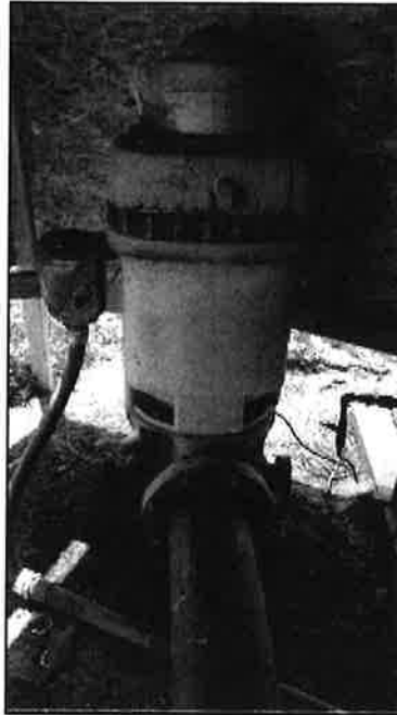
Figure 1: Well 1 75-hp vertical turbine.
