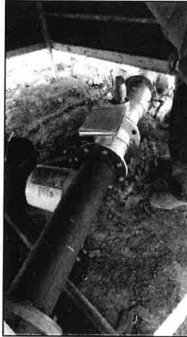
Figure 3: Discharge pipe of Well 1 showing flowmeter location.
