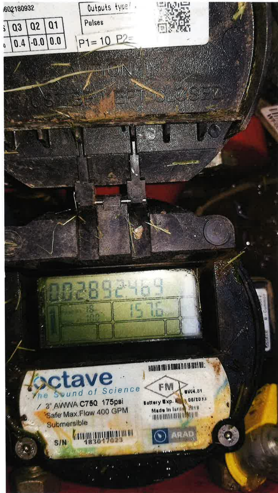
Figure 1: High flow rate on meter 157.6 gpm
