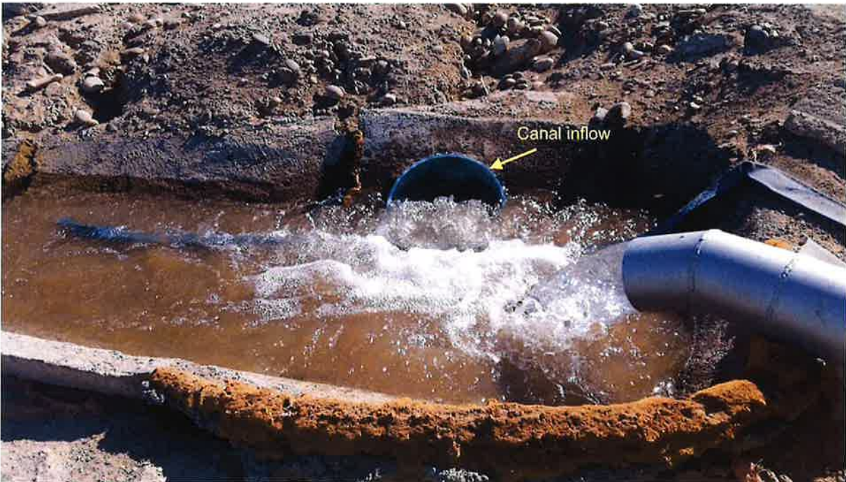
POD to ditch on north eastern edge of POU.
