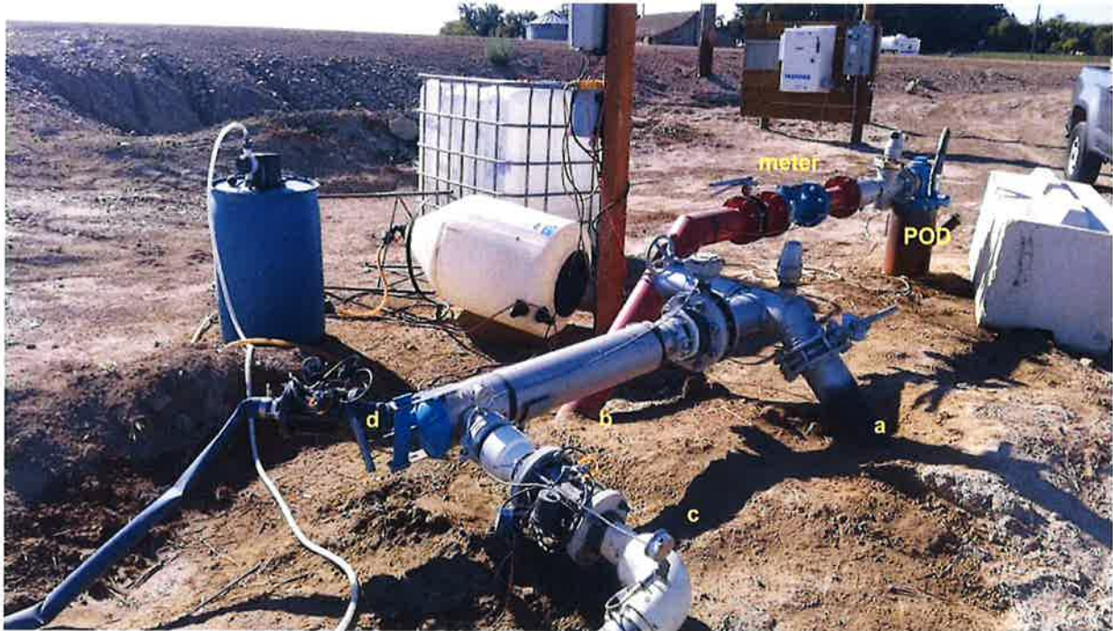
Point of diversion, metal tag D0071743. a) buried pipe that distributes water to NW-SE trending ditch in middle of the parcel b) Pipe to ditch c) Hose line to drip irrigation on NE field d) Hose to ditch.
