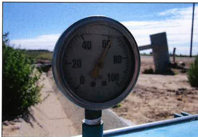
Figure 3: Pressure gage on pipe after booster pump (reading ~62 PSI).
