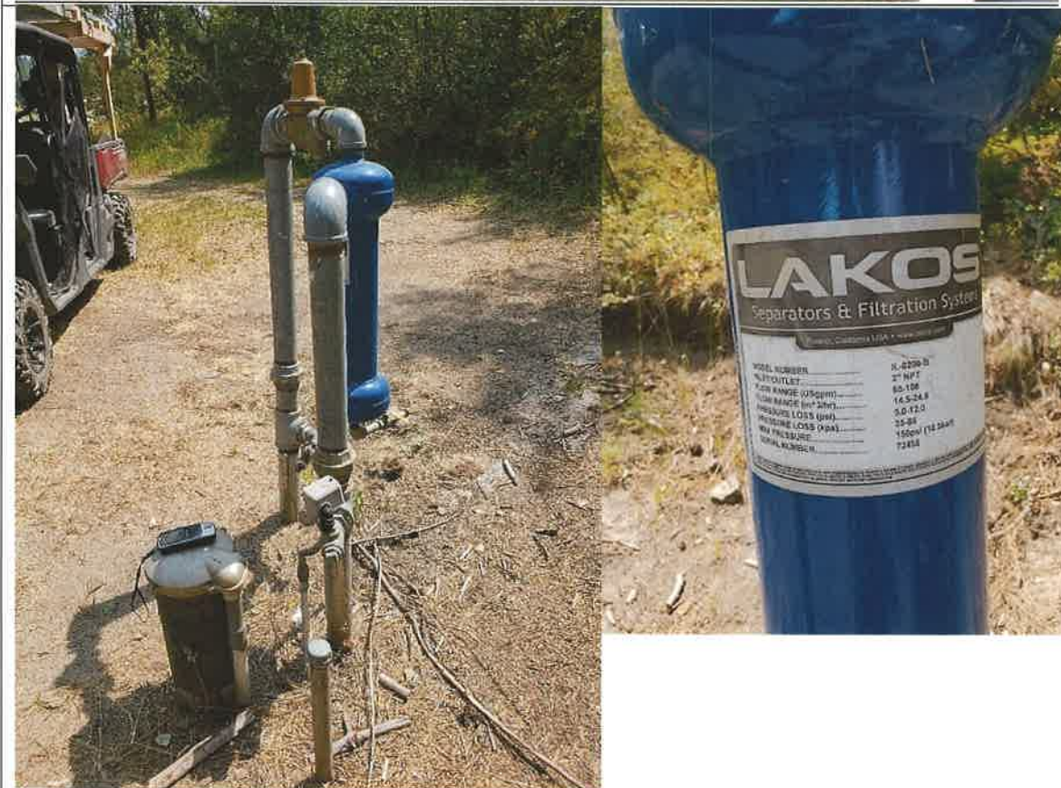
Figure 2. Well head with sediment filter. Sediment filter specification's showing associated flow range and pressure losses.
