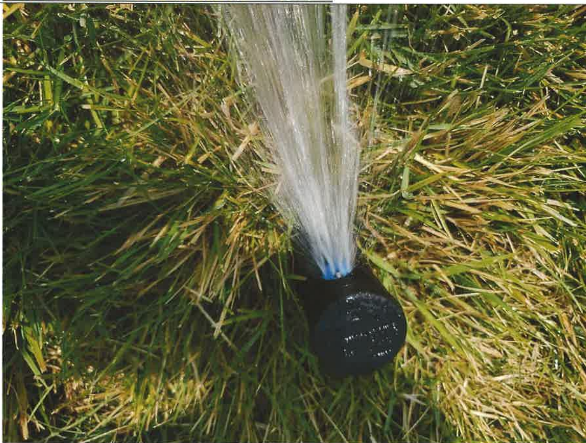
Figure 6. Nozzles were blue, number 9 with a 25° trajectory. According to manufacturer specifications for an operating pressure of 35 psi, discharge would be 4.2 gpm per head.
