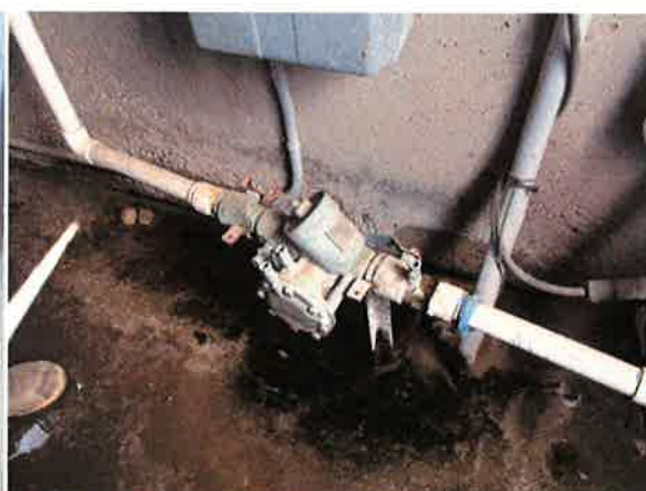
Backflow preventer inside re-use pump room
