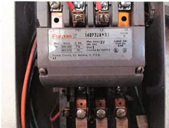
Inside pump power box for Well 7 1/2 HP
