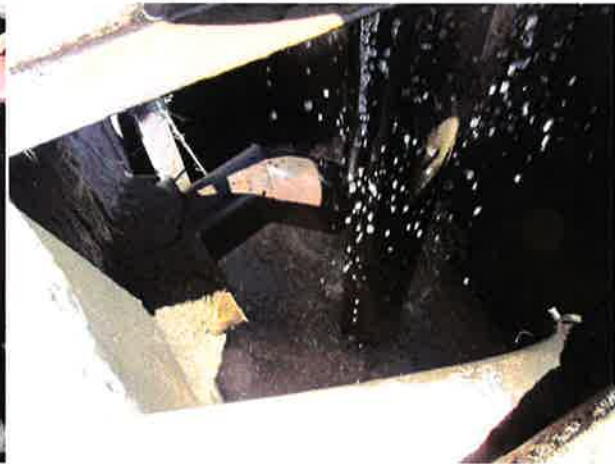
Inside irrigation box
