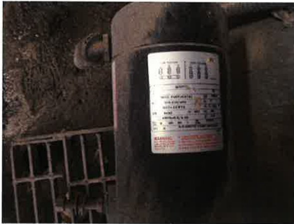
2 ea 2 hp pumps from re-use tank to stock-yard and barn
