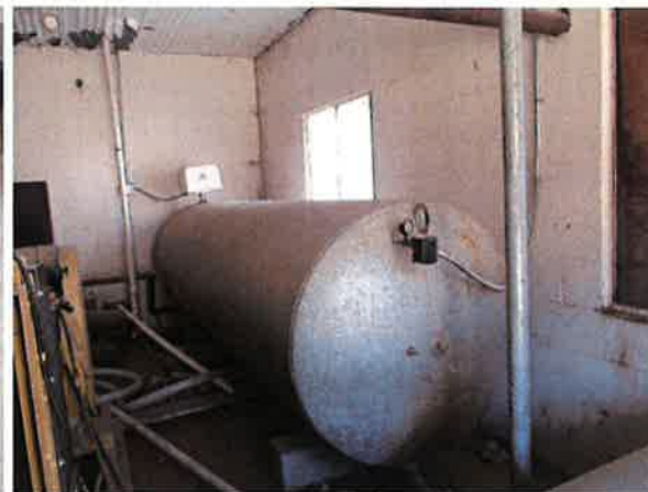
Pressure tank 42 inch X 143 inch
