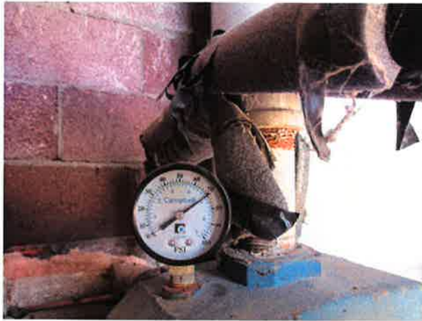
Grundfos pump not running maintaining 71 PSI
