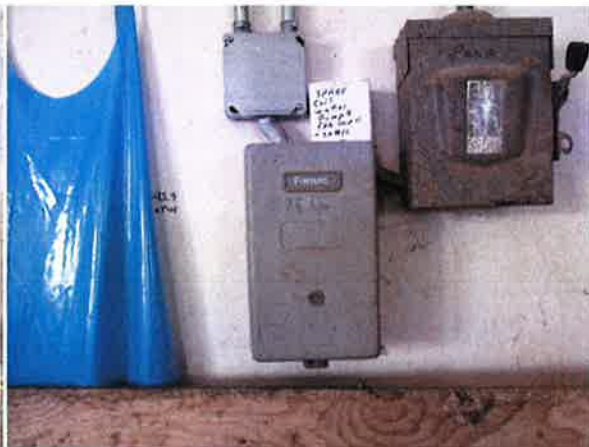
Pump power box
