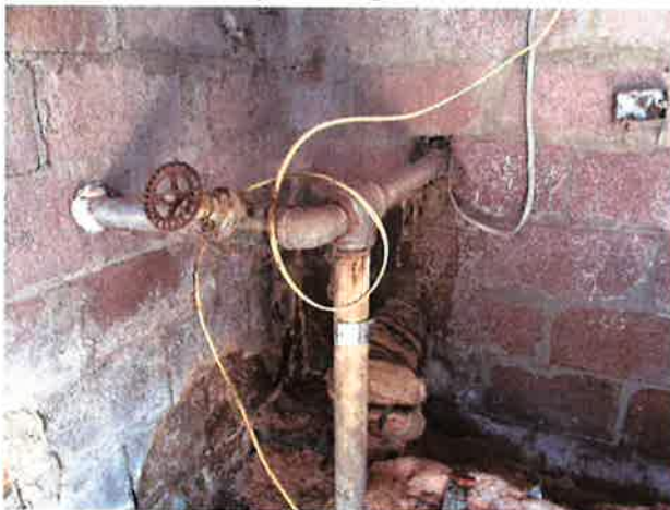
Control valve for this well
