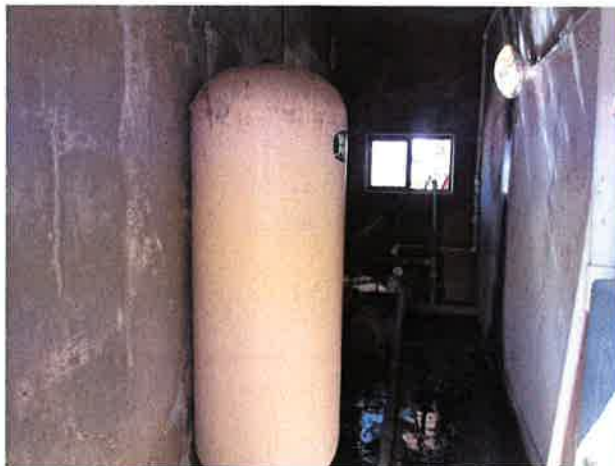
35 gal pressure tank in reuse tank pump room
