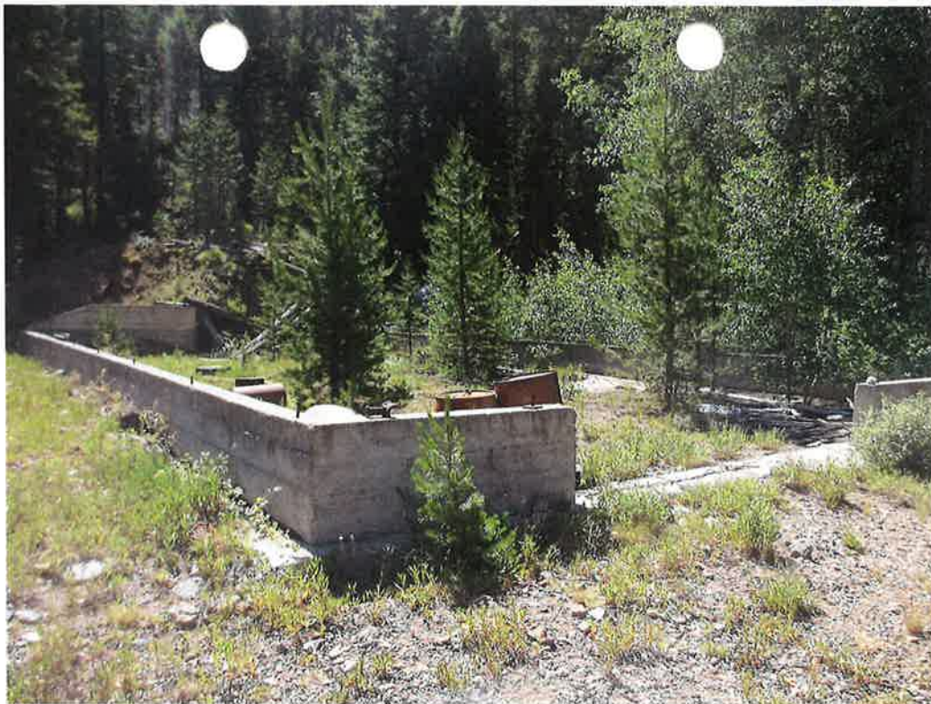
Remnants of the ore processing facility which collapsed from winter snow accumulation.
