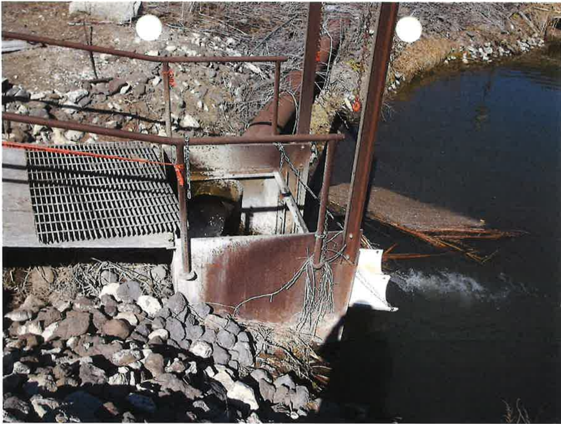
Return water from factory dumps into diversion channel before entering Rock Creek
