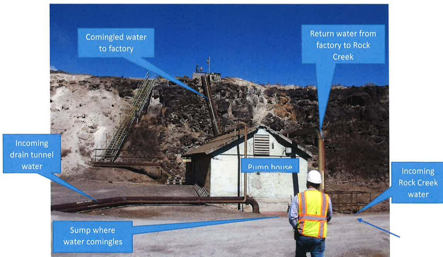
Pump house and associated piping
